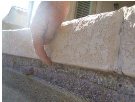
Horizontal crack in pool above steps
