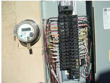
Interior of the electrical service panel
