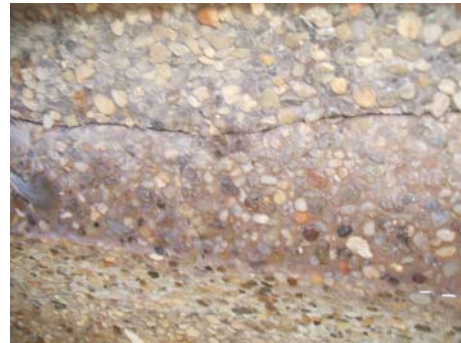
Close up of the horizontal crack
