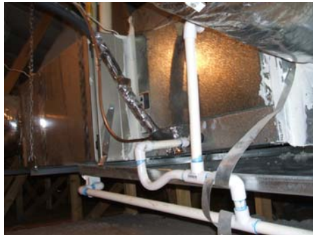
Heat Pump/air handler in the attic
