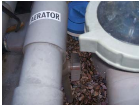
Aerator/general view of pool piping
